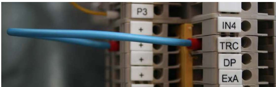
Electrical jumper for the time counter
